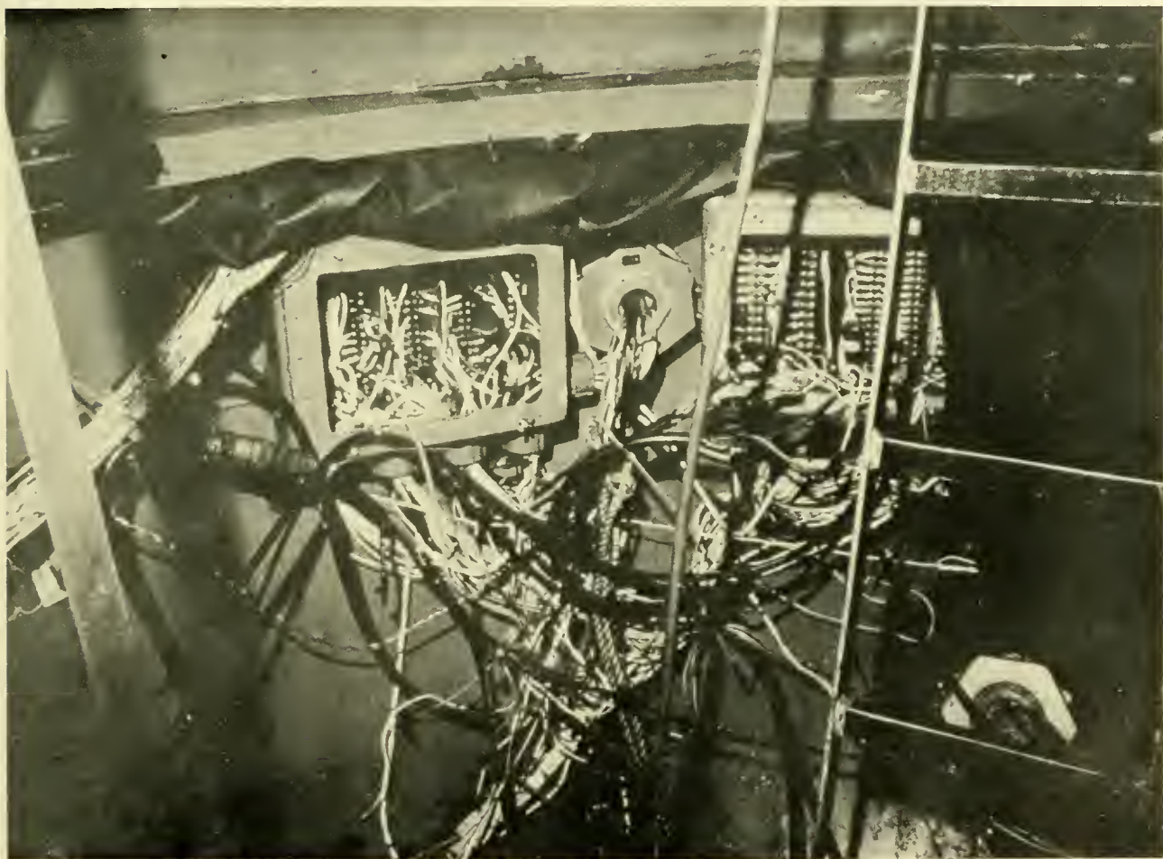
Fig 7.42 ALUMINAUT's internal junction boxes. (NAVOCEANO)
