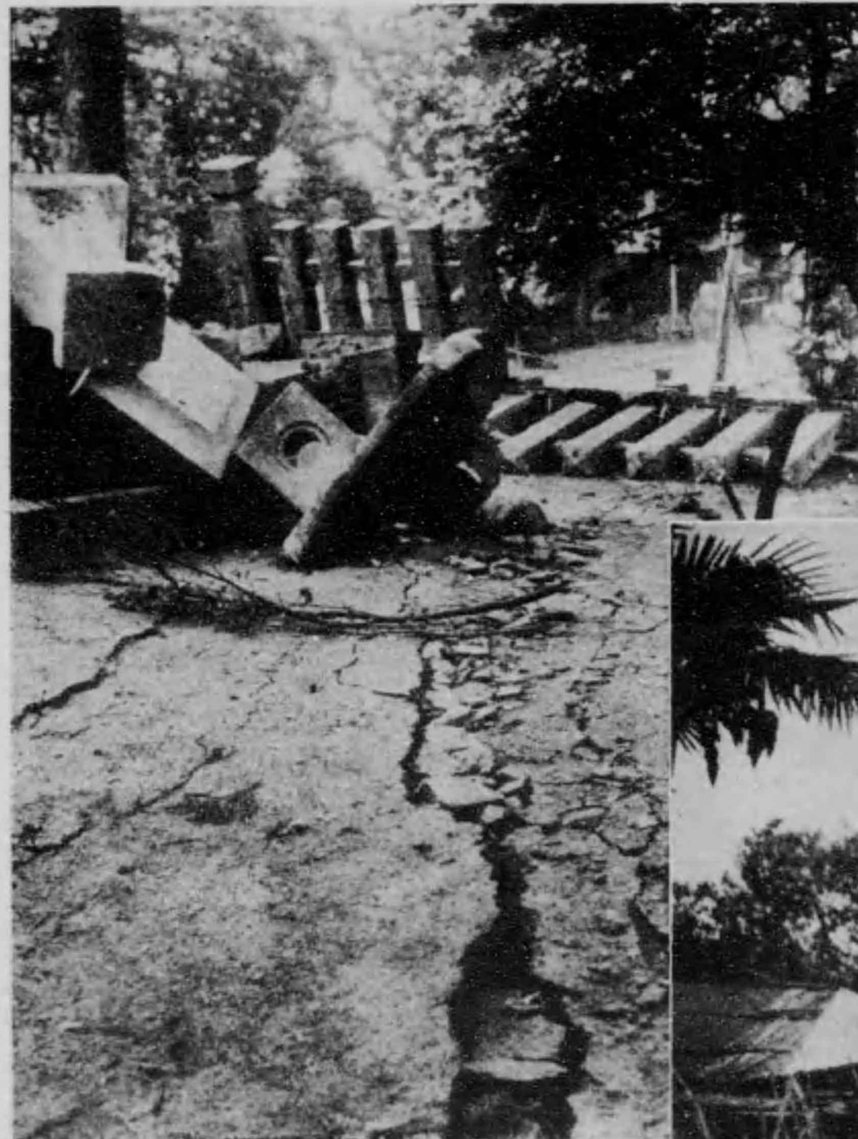
裂龜の内境社神吉日岡豊 Cracks caused by the earthquake. (Hiyoshi shrine, Toyo-oka)
