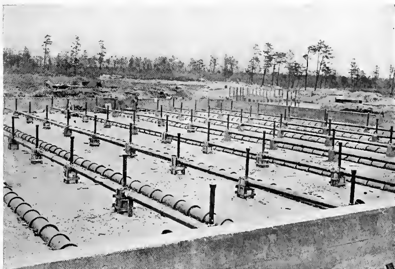
Fig. 44.—The sprinkling pipes and underdraining tiling of the stone bed of a sewage disposal plant ready to be covered with stone.
