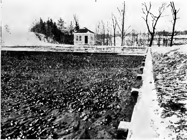
Fig. 50.—Stone bed of a sewage disposal plant.
