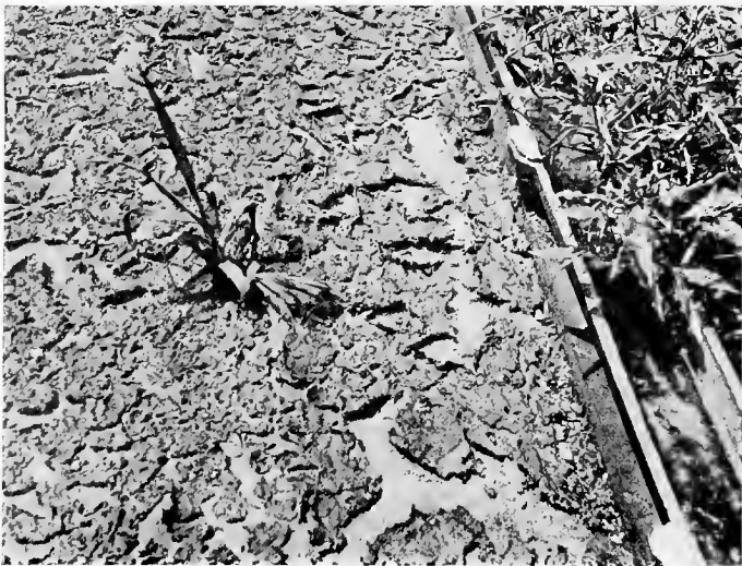
Fig. 49.—Dried sediment on the surface of a sand filter of a sewage disposal plant.
