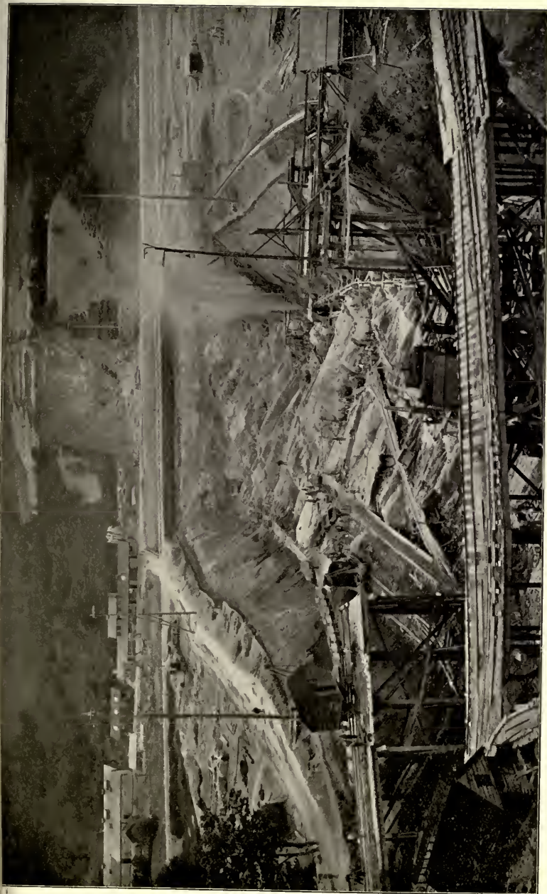
By permission of G. F. Deacon, C.E. No. 1. THE VYRNWY DAM—EXCAVATING THE TRENCH ACROSS THE VALLEY OF THE RIVER VYRNWY.
