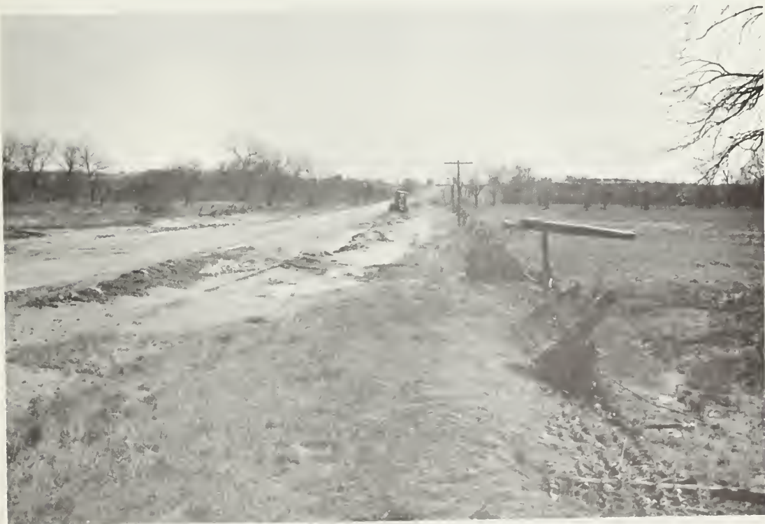
Damages occur frequently to roads and fences.
