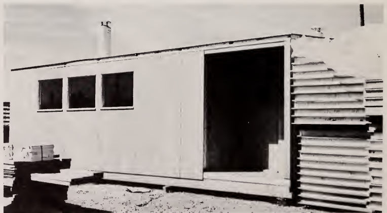
Complete except for painting, a two-bedroom unit assembled in the Muttart yard is surrounded by sections of similar homes ready for crating.
