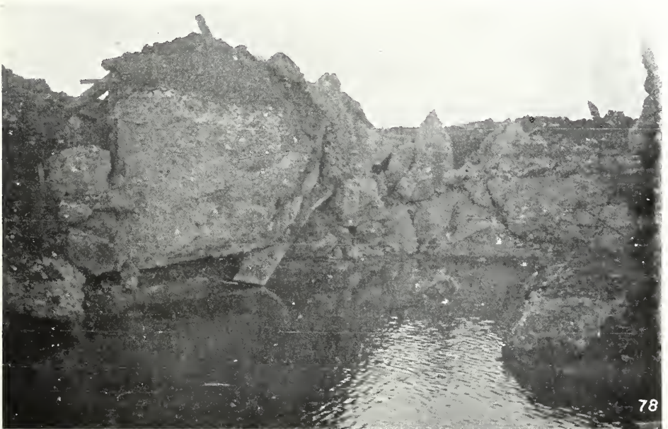
78. This one went off. The ruin here was once a mighty concrete machine-gun nest
