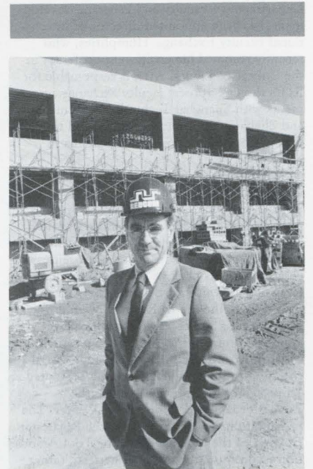
Hard hat area...RIT President M. Richard Rose, last week, reviewed construction of the new Center for Microelectronic and Computer Engineering, wearing a hard helmet presented to him by RIT alum Klaus Gueldenpfenning, president of Redcom Inc. Gueldenpfenning is a 1974 graduate of the College of Engineering and completed his MBA at RIT in 1977.
