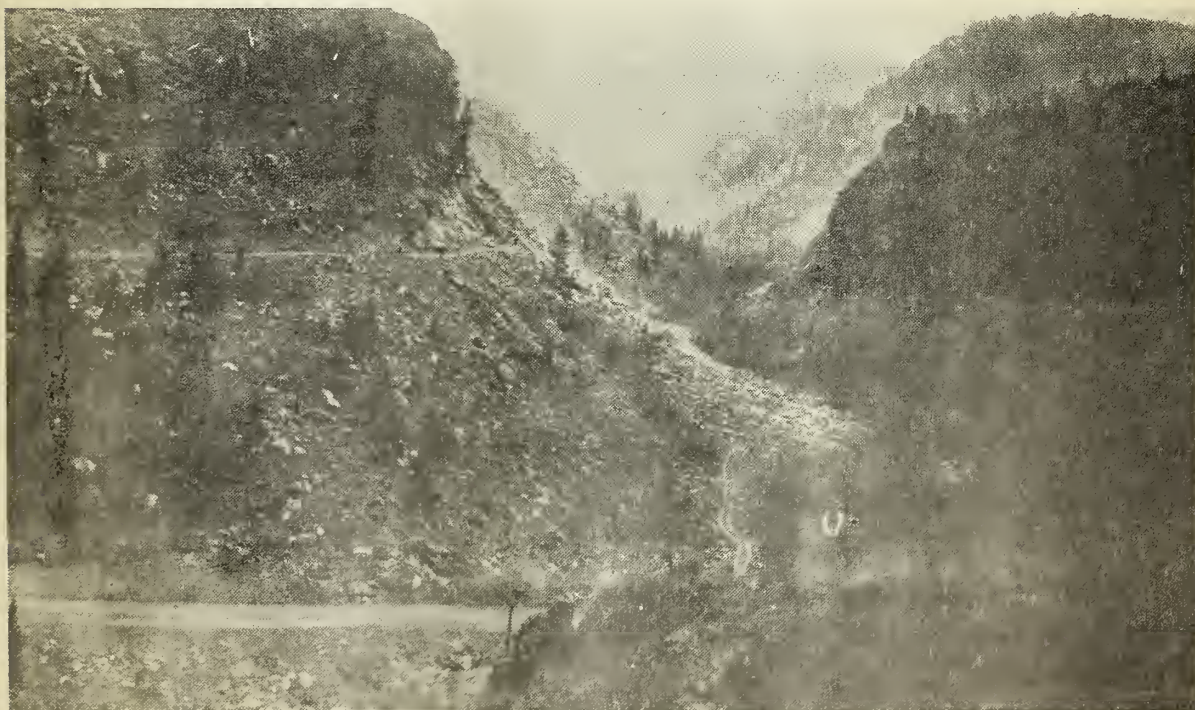
Figure 2-B. - After the smoke cleared away - cliff removed to a height of 135 feet and the old road blocked with rock fragments.
