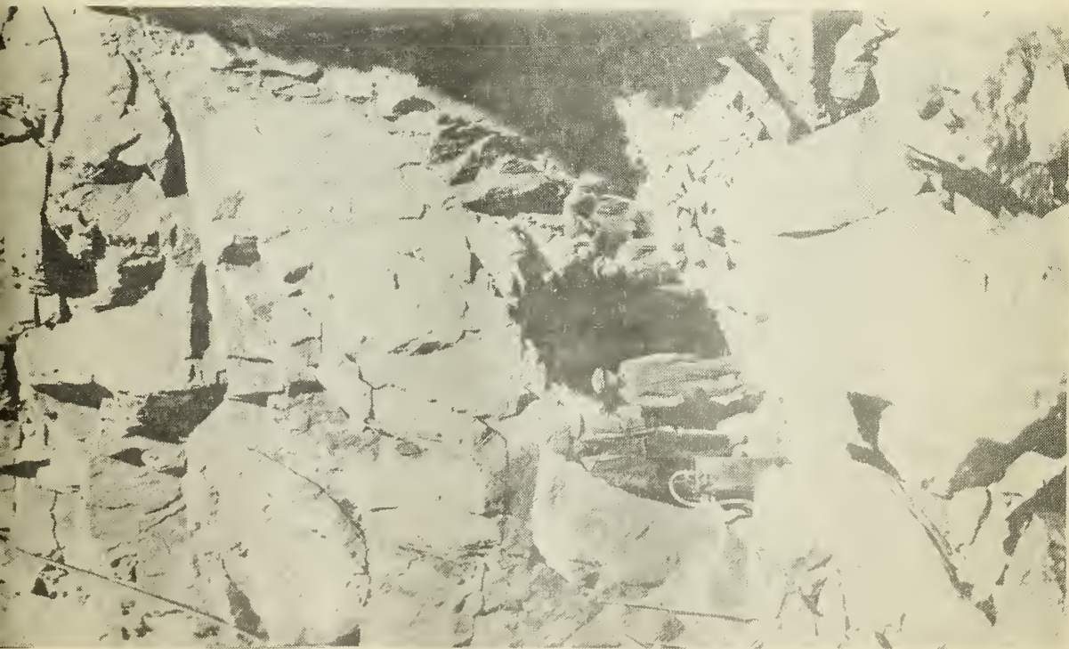
Figure 1-A. - The portal of the upper tunnel. The rope in the upper left corner of the picture was used by the workmen in going to and from the work.
