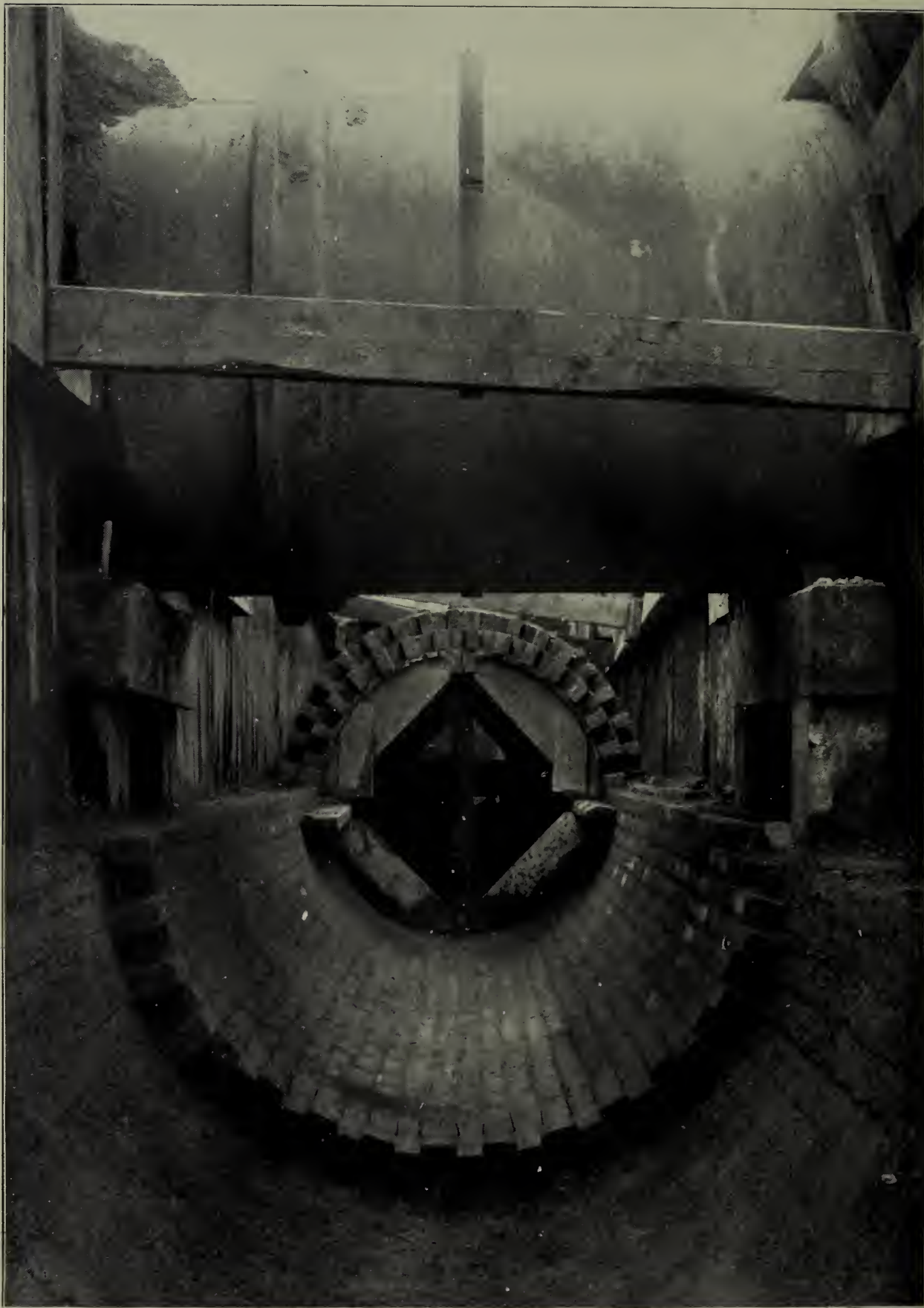
MYSTIC AVENUE STORM DRAIN, 50 INCH, Forbes Co., Boston. AT CROSSING WITH 48 INCH METROPOLITAN WATER MAIN.
