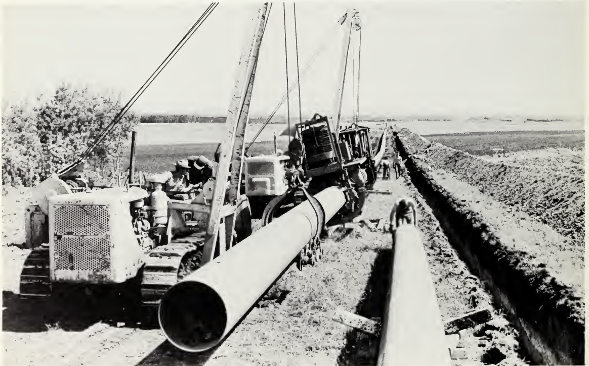
A network of pipelines, originating in Alberta, carry oil and gas as far east as Port Credit, Ontario, and as far west as Vancouver, British Columbia.
