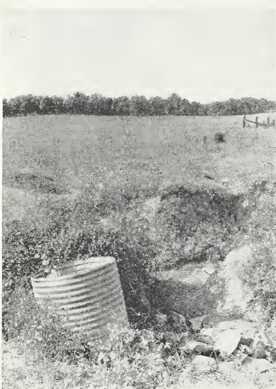
FIGURE 33.—A cistern sink near the center of a large basin 2 miles east of Irvington. Gullies about 6 feet deep were beginning to spread outward in several directions. In order to hold the water temporarily and check the gullies a 24-inch culvert pipe 8 feet long was placed in a vertical position in the sink. Rocks and brush have been piled around the pipe.
