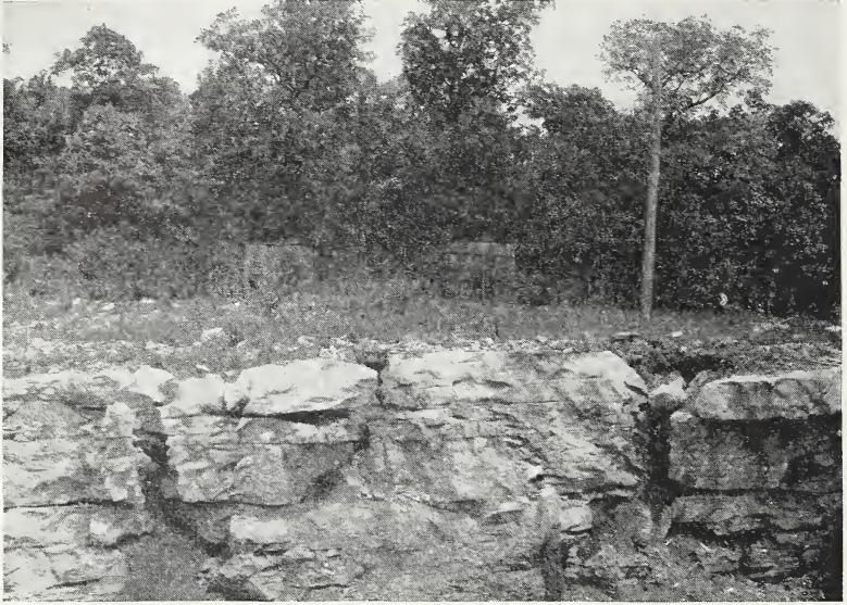
FIGURE 5.—Limestone bedrock and the overlying soil in a fresh road cut, 4 miles south of Monticello, Wayne County. Most of the soil was removed by erosion before the road was constructed. Note the fissures in the limestone partly filled with soil.
