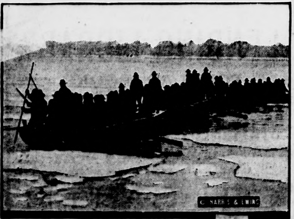
Abundant ice on the Potomac river has given engineer troops in training near Washington an excellent opportunity for overcoming obstacles. This picture shows "pontooners" breaking the ice preparatory to building a bridge.
