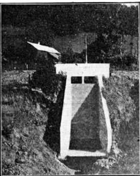
FIG. 2.—Road culvert and concrete drop inlet built at great expense to prevent gully from crossing the highway. It is shown partly undermined and later was washed out. Near Alma, Wis.
