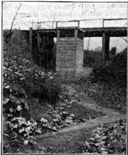
Fig. 28.—Drop inlet and box culvert. Plan shown in Figure 29. The old wooden bridge is to be replaced by an earth fill
