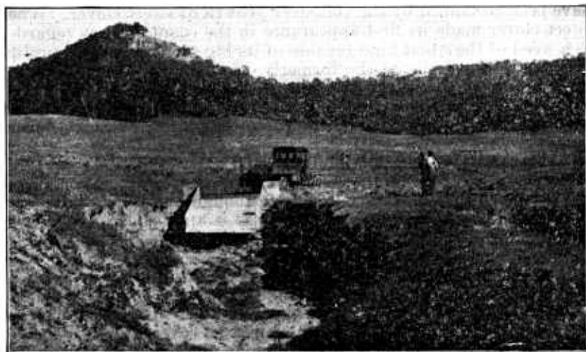
FIG. 10.—Water conducted into head of gully by levee and a sheet-metal flume, the left-hand levee not yet built; brush and stone to be placed at the lower end of the flume. Near Alma, Wis.
