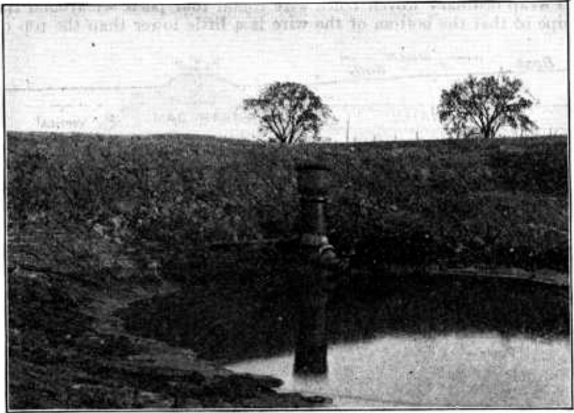
FIG. 24.—Vertical inlet pipe newly constructed, showing hopper pipe on top and end of T plugged with vitrified clay stopper cemented in the pipe. Near Marshall, Mo.
