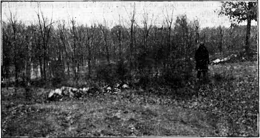
FIG. 18.—Upper side of a loose rock dam across a gully. A fill of 2 feet has occurred where the man is standing. Near Franklin, Tenn.
