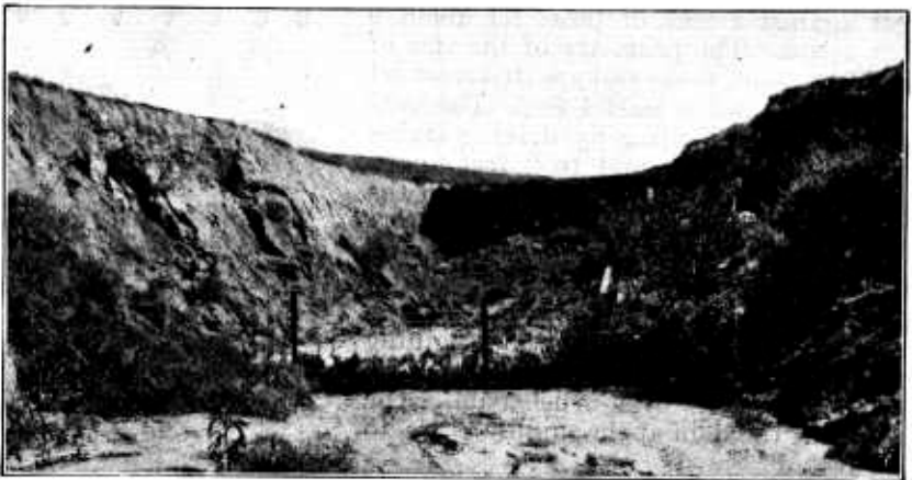
FIG. 15.—Newly constructed woven wire fencing dam built to control erosion at head of gully. Near Alma, Wis.
