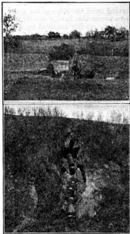
FIG. 25.—Results of water seeping along outside pipe through a dam
