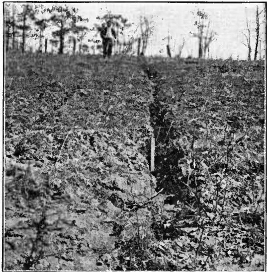
FIG. 5.—The beginning of a gully down a hillside caused by the passing of a wagon once down the slope, if not controlled, destined soon to be a large gully. Near Jackson, Tenn.
