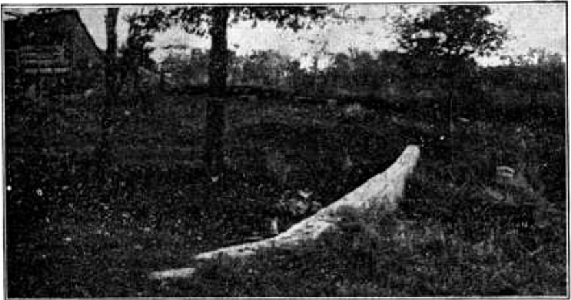
FIG. 19.—Masonry dam built across a gully draining over 1,000 acres. This dam extends well into the banks and is lower in the middle than at the ends. Near Kansas City, Mo.
