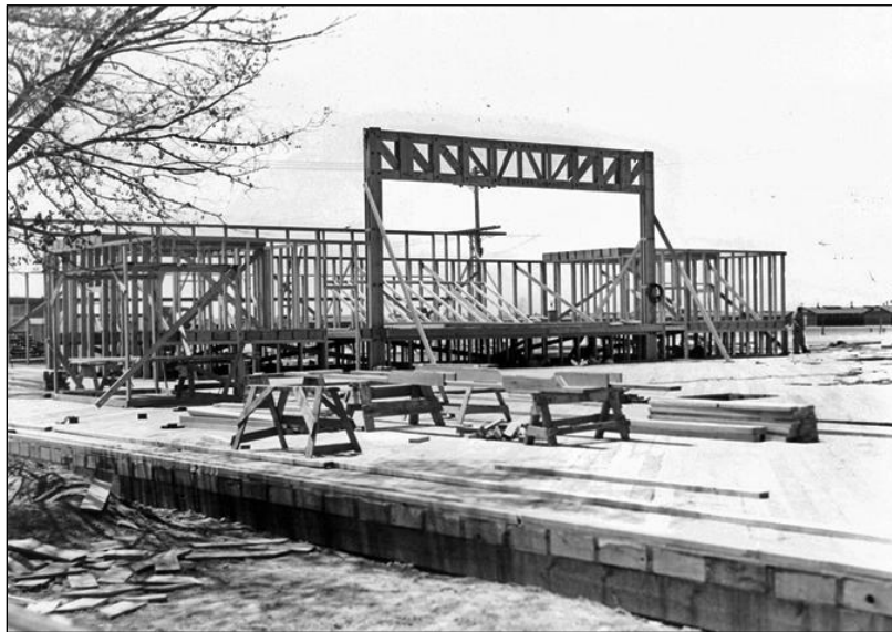
The first truss is installed for the high school at the Topaz Relocation Center. WRA photo by R. Bankson, July 1943 Courtesy of the U.S. National Archives and Records Administration
