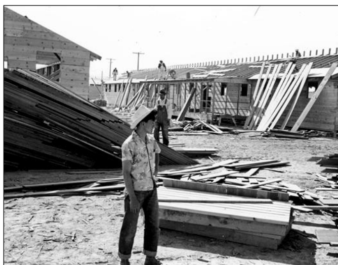
Larry Orida watches construction of the hospital at the Poston Relocation Center, Site I. WRA photo by Fred Clark, May 12, 1942 Courtesy of the U.S. National Archives and Records Administration
