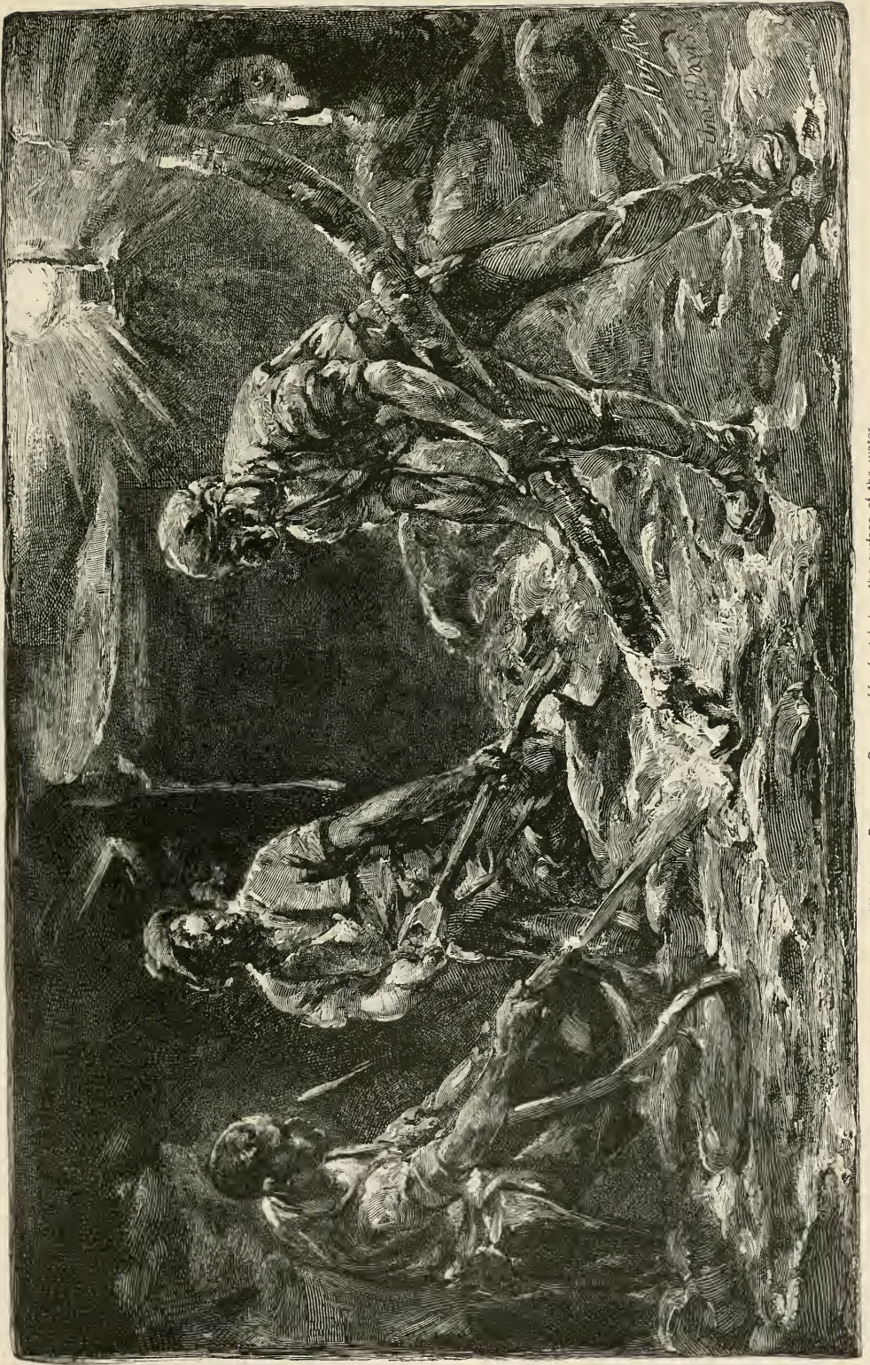
At Work in a Pneumatic Caisson—fifty feet below the surface of the water.
