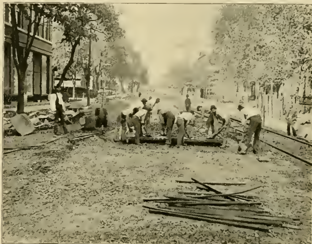
All Steel Track, Terre Haute. Third Process, Laying the First Eight Inches of Broken Stone.
