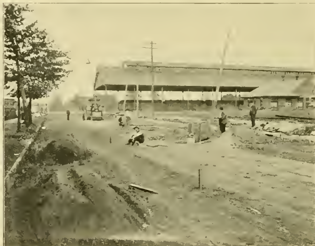
All Steel Track, Terre Haute. First Process, Rolling the Roadbed after Excavation.
