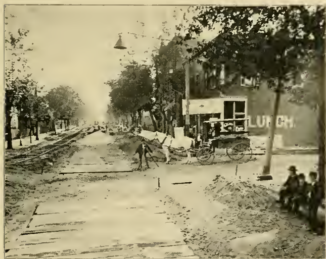
All Steel Track, Terre Haute. Second Process,—Preparing to Receive the Broken Stone. Setting the Stakes.
