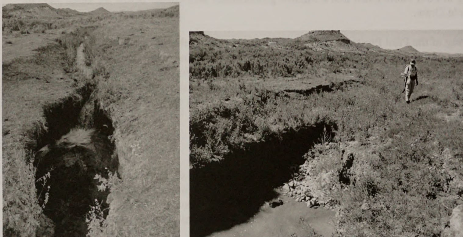
Figure 1: Pictures of headcut during the first two years (2001-2002). The picture on the left shows the change in velocity that down cuts the headcut and allows it to migrate upstream with small discharges. After the initial vertical adjustment the headcut widens with bank sluffing shown on the right. Note the current position of the headcut is in the sagebrush shown in the background.
