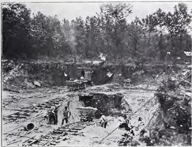
FIG. 13.—Excavation in white clay near Holly Springs, Pa. The overlying quartzite outcrops at the base of the slope seen in the distance.
