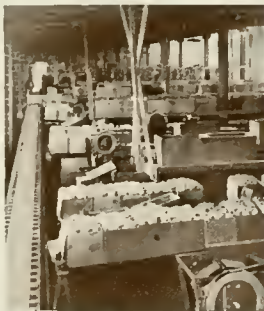
Portion of Standard System installed in the packing plant of the Peshastin Fruit Growers' Assn., Peshastin, Wash.
