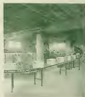
Spiral chute delivering boxes on a gravity roller conveyor to shipping department for storage or transportation.
