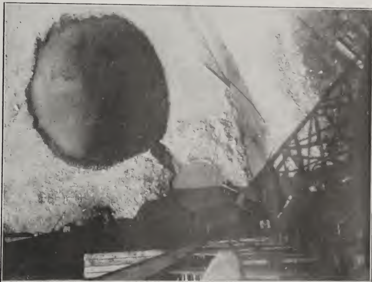
Fig. 34. Photograph of the mud sump taken from the top of the derrick on Selby-Cisler well, Ewing No. 6B.
