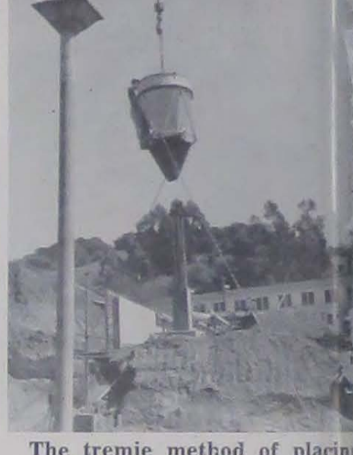
The tremie method of placing concrete under water in piers employs upright pipe into which concrete is poured. The workman lifted high above the excavation, his bucket loaded with concrete, makes many trips before form is filled.
