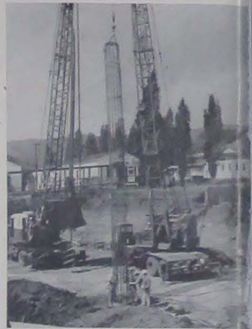
Here, reinforcing steel for concrete pier is being set in place. More than 200 piers are already in. The deepest will be 77½ feet.
