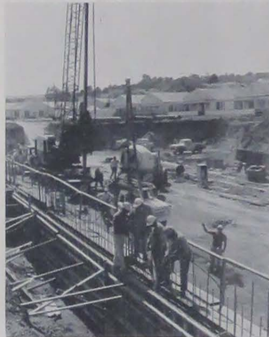
In this picture workmen are pumping concrete into the wall form, much as one squeezes toothpaste from a tube. The man at right helps position the tube.
