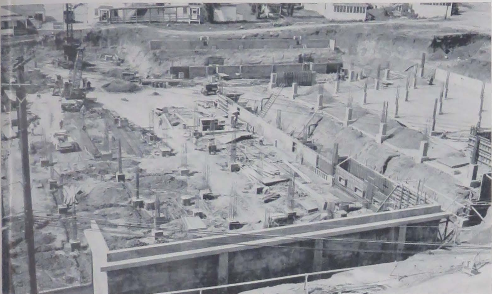
THE BIG HOLE —first step toward the new Oak Knoll—becomes more interesting each day as workmen from Huber, Hunt, and Nichols of Santa Clara go about their gigantic task. This overall view shows, in left foreground, the crawl space under the first floor. Here, in addition to the steel-reinforced concrete piers now clearly visible, the heating and plumbing ducts and pipes for the nine-story building will be located. At right, the crawl space under the second floor may be seen. Barely visible in the right lower corner are forms for the foundation of the new cobalt therapy unit, whose walls will be 23½ inches thick.
