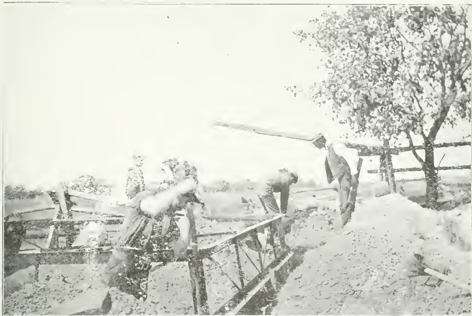
Footings being set by means of Special Template, to which the Four Footings are bolted.
