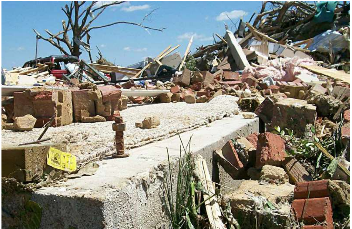
Looking south, protruding anchor bolt (washer/nut intact) from slab with base plate ripped away. No standing walls, just rubble. Debarked hardwood trees in background. Photo location Smithville, MS. (Photo: WFO Memphis)
