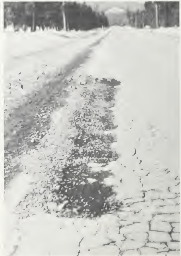
Figure 7—Typical alligator cracking resulting from heavy haul during weak pavement conditions.
