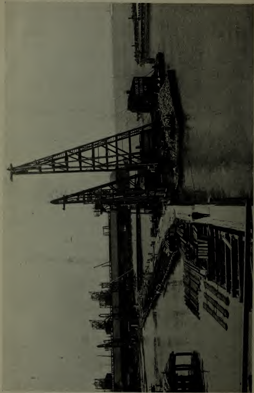
Section 9 of the seawall in process of construction. Flooded area to the left is now being filled in to make seawall lots.
