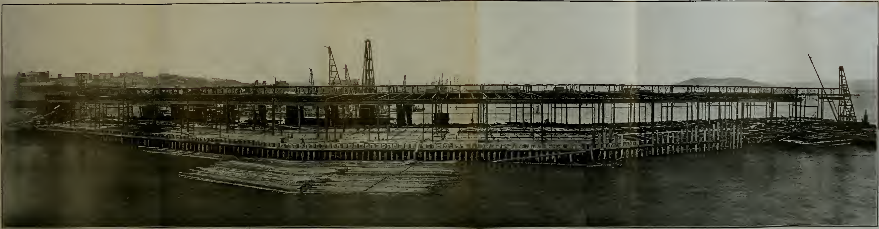
PIER 38 AND SHED IN COURSE OF ERECTION, SHOWING CHARACTER AND PROGRESS OF NEW CONSTRUCTION.
