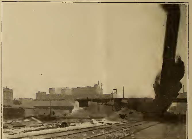
Clearing ground for Chicago's new Union station. Copyright 1915 by Hearst-Selig News Pictorial.
