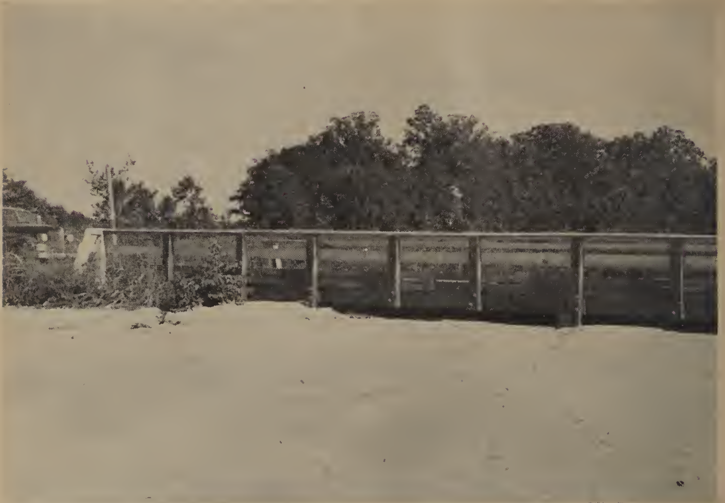
PLATE 4. Stream bed under highway bridge completely blocked with sand. Brown loam physiographic area.
