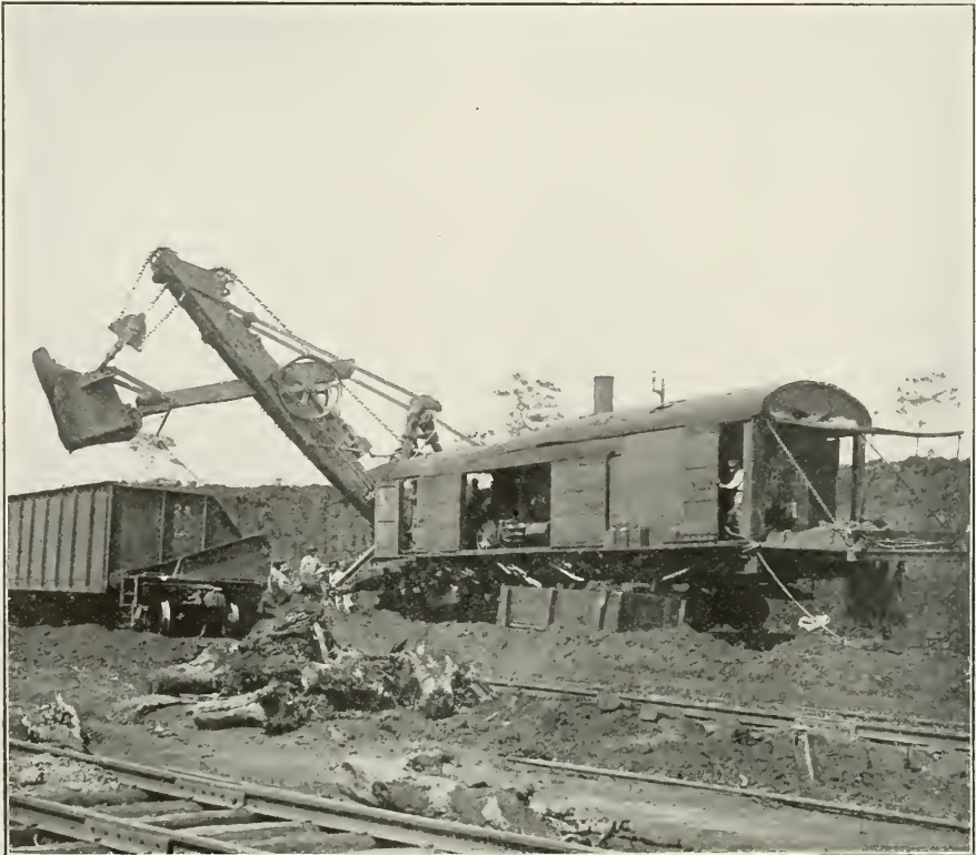
Steam shovel at work in the mines of the Spanish-American Iron Co.
