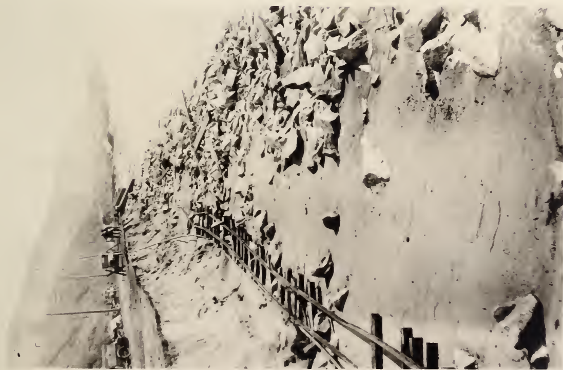
FIGURE 6. - DAMAGE TO STATE-BUILT MIDDLE SECTION DONE BY STORM OF FEBRUARY 11 TO 13, 1926. A WALL IS NOW BEING CONSTRUCTED AT THIS POINT.
