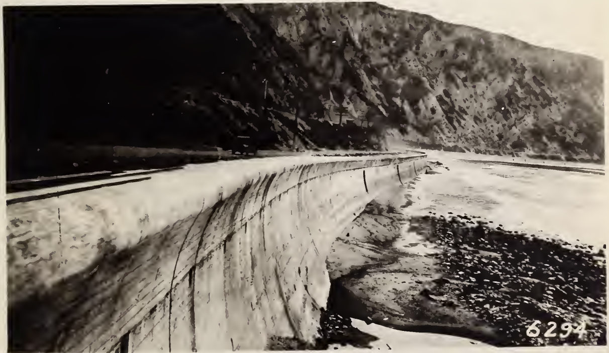
FIGURE 5. - SECTION OF THE COMPLETED WALL, BACK FILLING AND TEMPORARY CRUSHED ROCK SURFACE.
