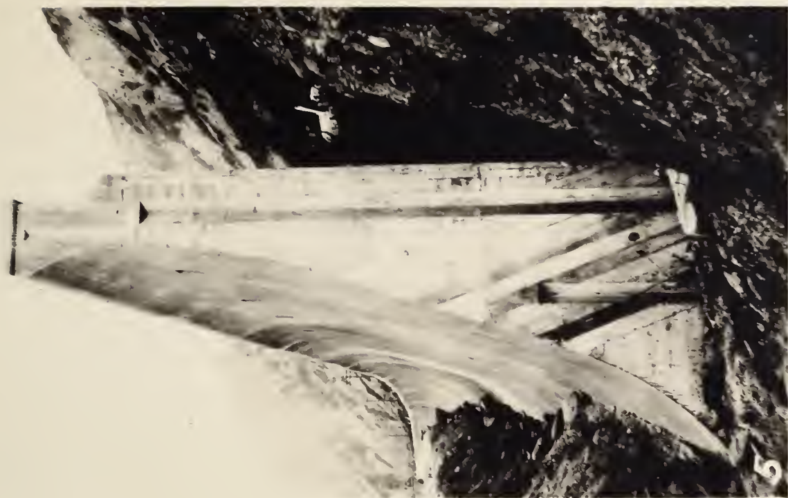
FIGURE 7. - END OF WALL SHOWING KEYS AT THE CONSTRUCTION JOINTS. ORNAMENTAL STAIRWAYS FROM THE ROADWAY TO THE BEACH ARE UNDER CONSTRUCTION AT THE ENDS OF THE WALL.
