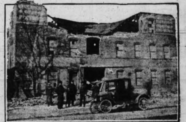
A tornado left scenes like this after it had swept through St. Joseph, Mo., inflicting $200,000 in property loss. This building had to be entirely rebuilt.
