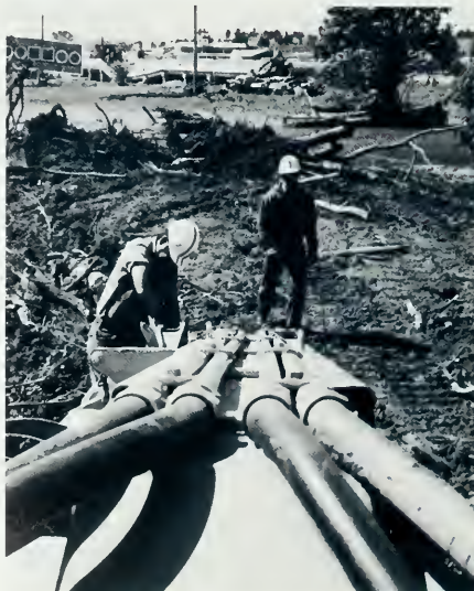
Northwestern Bell salvages remains of cable damaged by the Rapid City flood.
