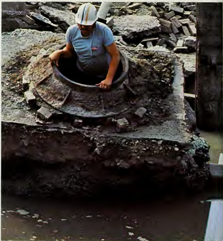
Manhole and telephone conduit lie above ground after flood washed away a Wilkes-Barre street.
