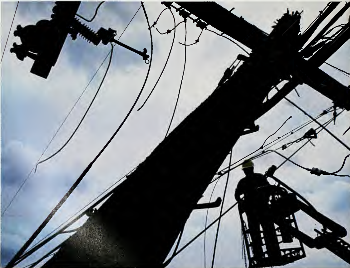
Restoring a critical communications link. Flood uprooted pole and left aerial cable in shreds.
