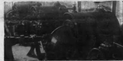
View of Generator Room.
