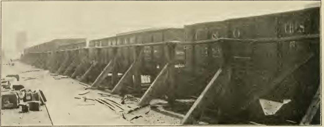
View of North Side of North Track Showing Elevated Runway Used by Rivet Burners and Backout Men
