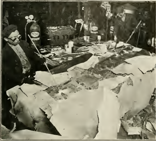
Fig. 3—Welding Defective Condenser Casting
