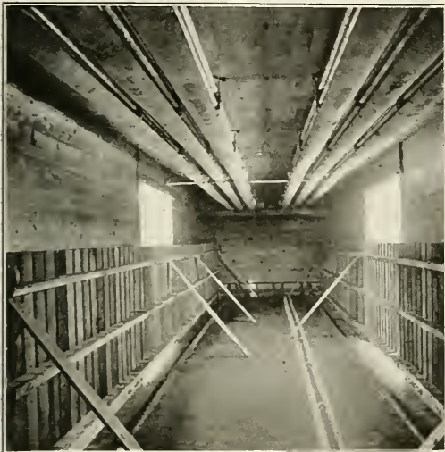
Fig. 17—Car with Overhead Brine Tanks, Showing Also Heater Pipes on Floor
