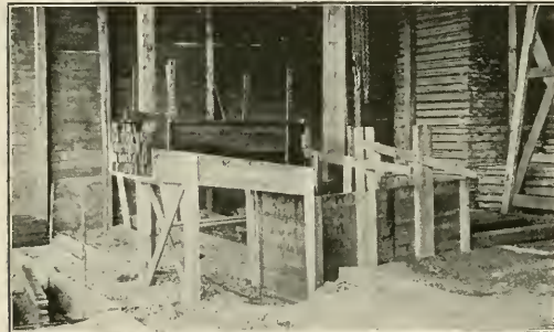
Small Tank for Creosoting No. 1 Common Yellow Pine Decking and Roofing; 250 to 400 Pieces Per Charge Immersed 30 Min.; Repairs Caused by Decay Already Reduced More Than 50 Per Cent
