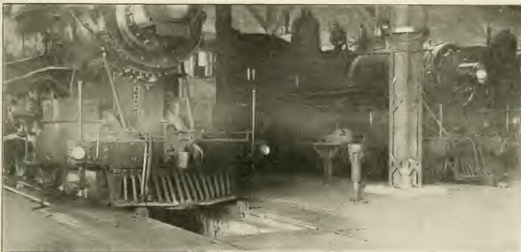
Boiler Washout Section, Showing Depressed Drains, Post Cranes, Etc.
