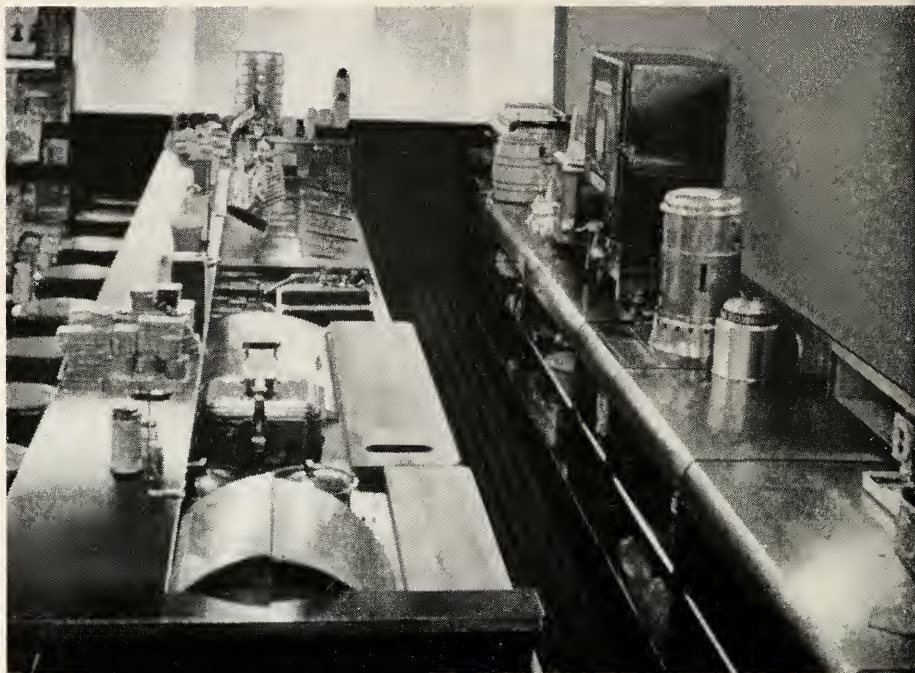
A recent installation of Bastian-Blessing Soda Fountain-Luncheonette equipment at Thomas Hogshead, Inc., Staunton, Virginia
