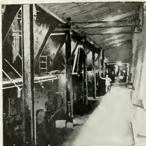
BOILER ROOM SHOWING COAL SHUTES.
