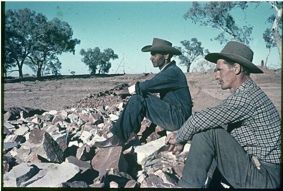
Work on the Stuart Highway (south of Alice), Northern Territory Public Works Department
