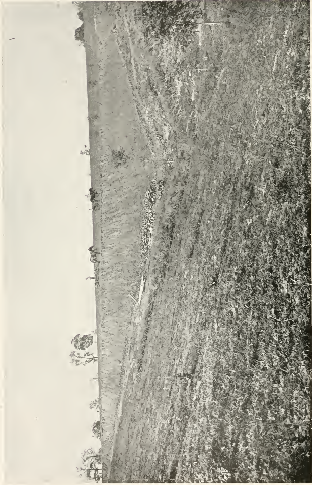
Courtesy U. S. Geological Survey. CONSTRUCTING AN EARTHEN RESERVOIR EMBANKMENT, COLUMBIA, MO.
