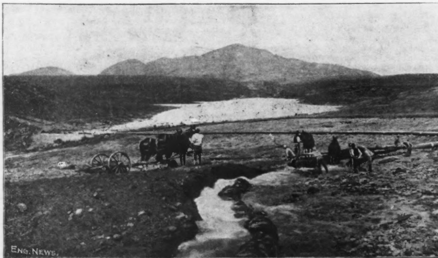
FIG. 2.—PROPER USE OF THE HYDRAULIC METHOD OF DAM BUILDING—LA MESA DAM, NEAR SAN DIEGO, CAL.
