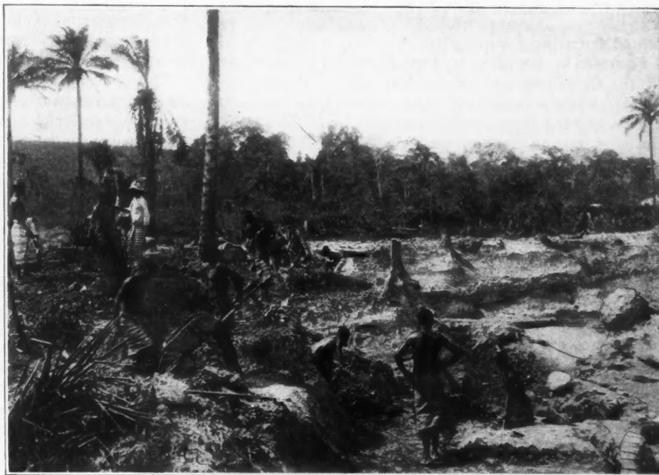
TAKING OFF OVERBURDEN IN THE GRAVEL PIT AT M'PESO, KASAI DIAMOND FIELDS
