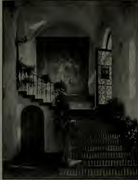
The simplest form of groined vaulting, decorative without ornament. In the H. H. Rogers house, Southampton. Walker & Gillette, architects
