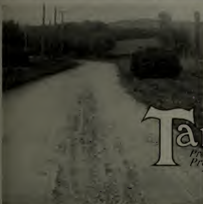
Forest Lawn Road, Florence, Neb., showing condition of road before the use of "Tarvia-X."
