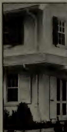
The drain pipe section is protected against damage from garden tools
