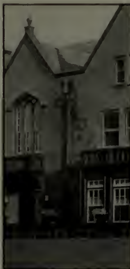
Where the leader head and downspout are made to serve a decorative purpose
