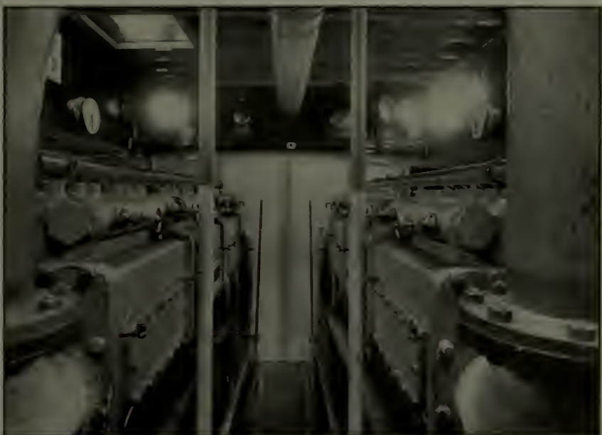
Engine room of a 100-foot cruiser. To effect a proper distribution of weights, the engines generally occupy the choicest position of a boat. These two six-cylinder motors develop 200 horsepower each
