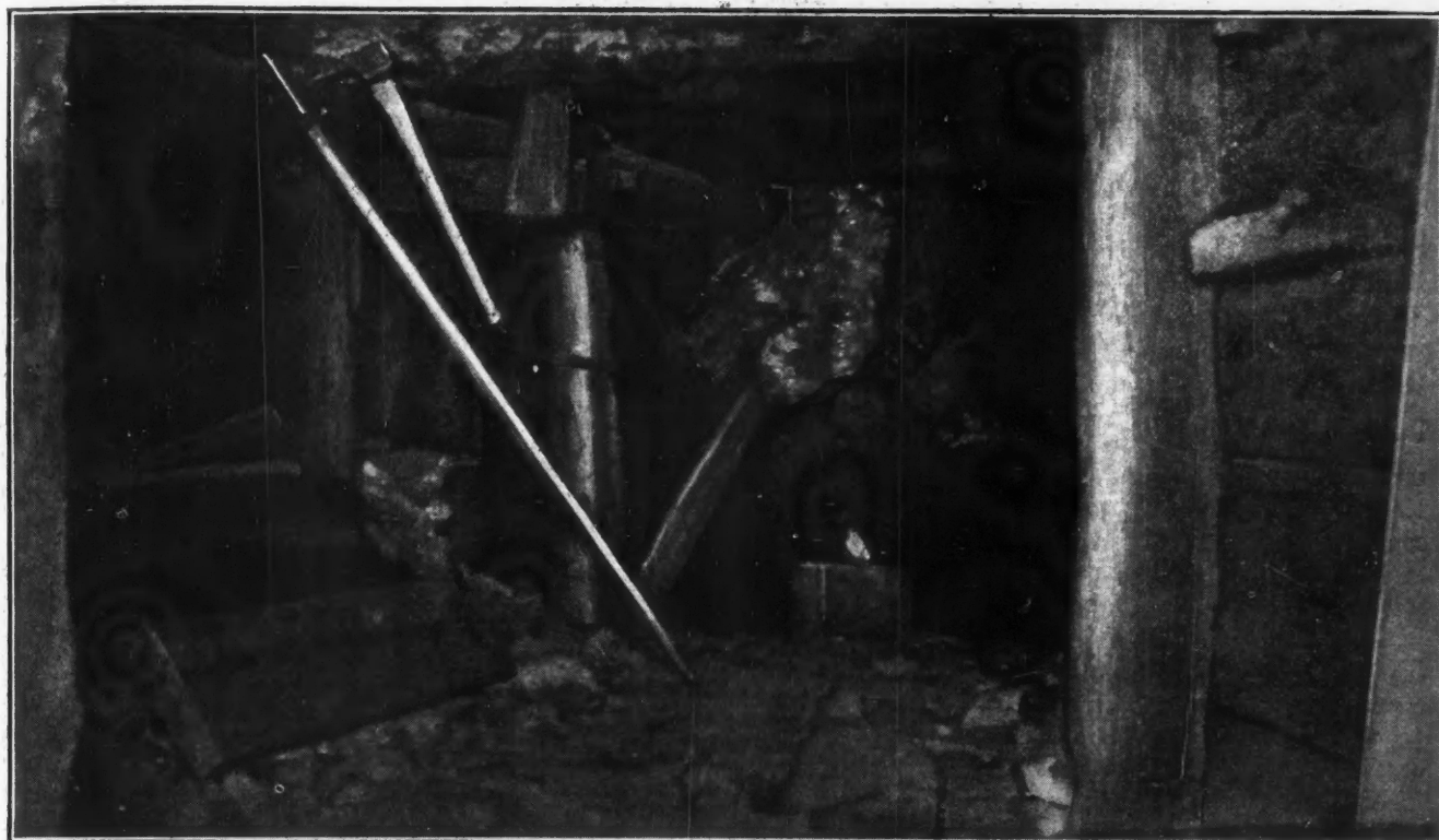
FIG. 1. TWO 16-FT. SPLICED STULLS FOR THE NEXT SET AHEAD IN THE CAVED PORTION OF A STOPE ARE TEMPORARILY SUPPORTED ON STRINGERS EXTENDED FROM UNDER THE CAPS OF THE SETS IN PLACE
