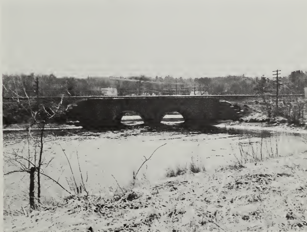
Ashland -- This Penn Central Railroad twin arch bridge at the upper end of Reservoir No. 2 acts as a bottleneck to major peak flood flows. (SCS photo)
