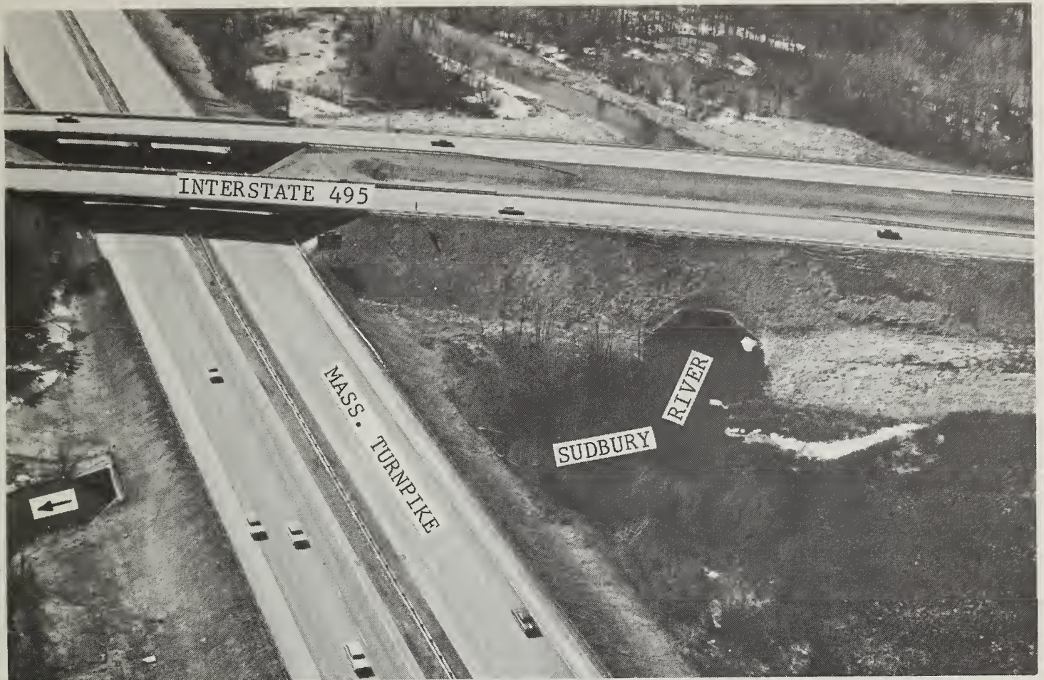
Westborough -- Hopkinton -- Major Interstate highway construction through Cedar Swamp with crossings over the Sudbury River. (W.R.C. photo)
