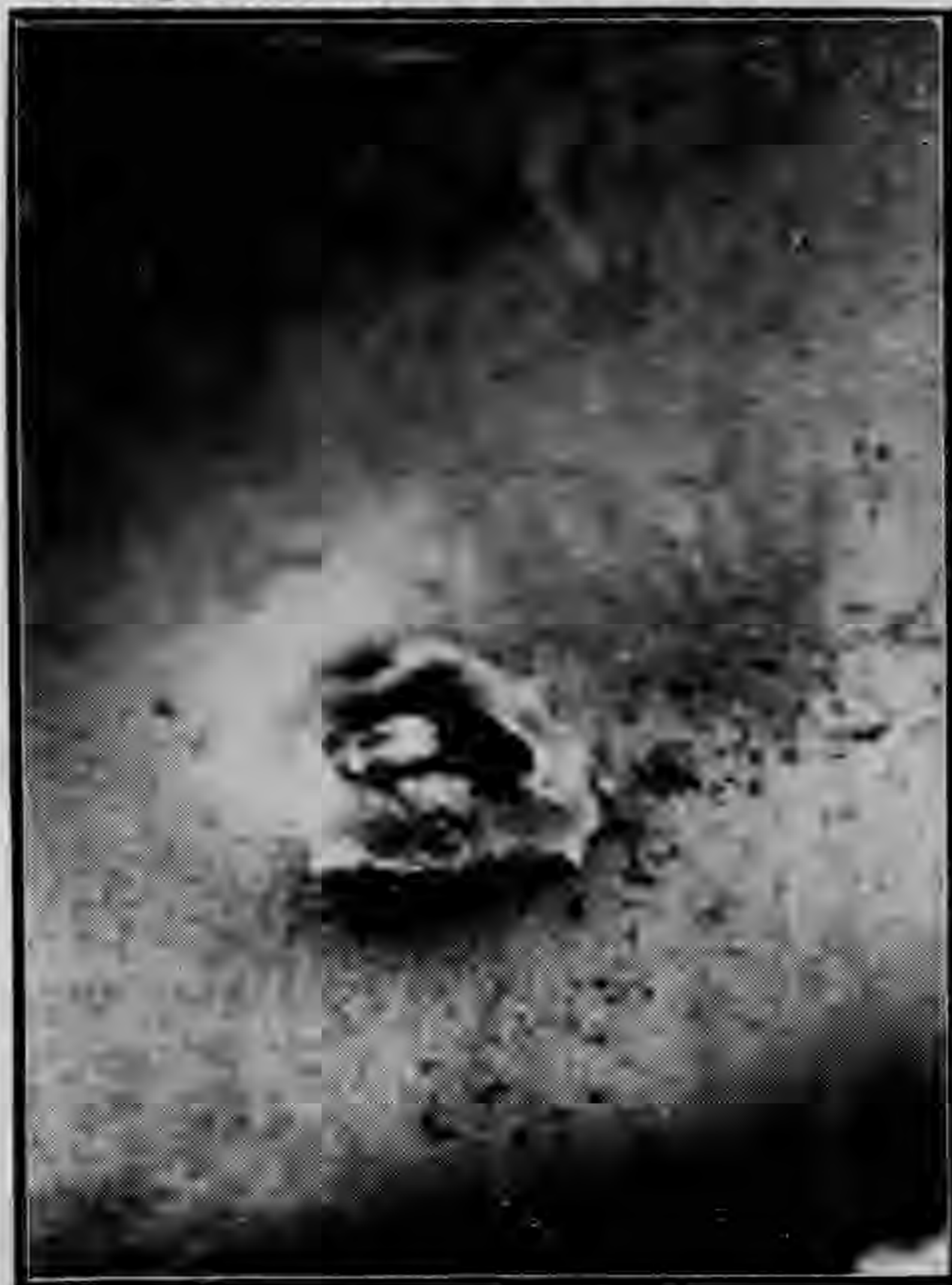
Fig. 4. A hole made in the steel plate on the side of the 3rd class coach No. 208 by a machine-gun cartridge. The shot penetrated through in an oblique way with the outside end higher than inside opening shewing that the shot was fired from above.
