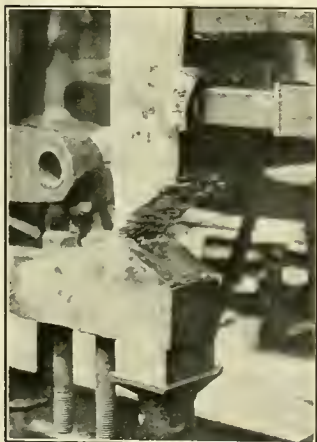
Broken Pedestal V'd out for Electric Welding
