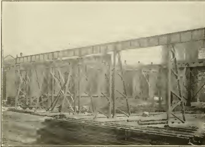
Runway for the Outside Traveling Crane
