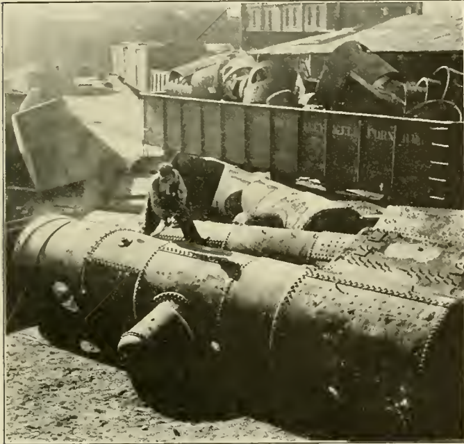
Old Boilers and Fireboxes Are Cut with the Oxy-Acetylene Burners Into Pieces Convenient for Handling
