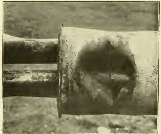
Superheater Tube Which Collapsed from the Effects of Improper Treatment in Welding
