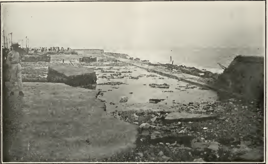
Section of the new seawall, several hundred feet in length, which was washed out during the storm of September 9th. This section is in front of Santa Clara battery on the road leading from Havana to Vedado. (Photo by American Photo Co., Havana.)
