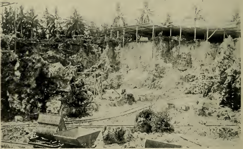
Ocean Island Phosphate Workings. Foreground: Most of the phosphate has been removed exposing the coral limestone pinnacles. Background: Phosphate deposit is intact and exists mostly in the form of gravel with occasional large boulders of phosphate rock.
