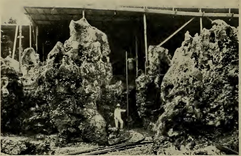
Ocean Island Phosphate Workings. Coral pinnacles after most of the phosphate has been removed. A few feet more phosphate available below rail level.
