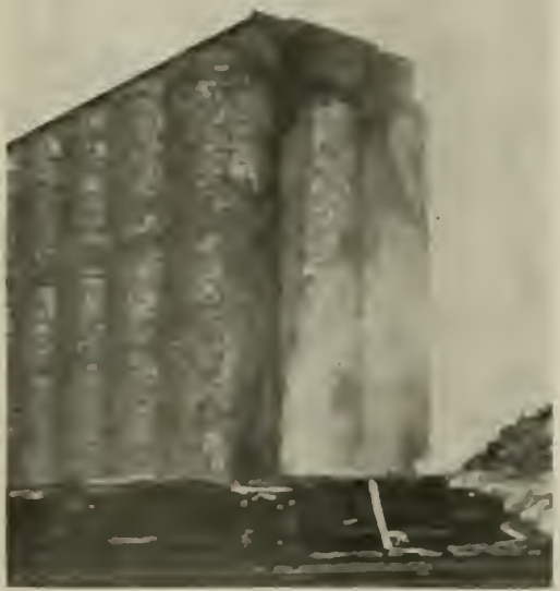
EFFECTS OF FIRE ON THE CONCRETE STORAGE TANKS
