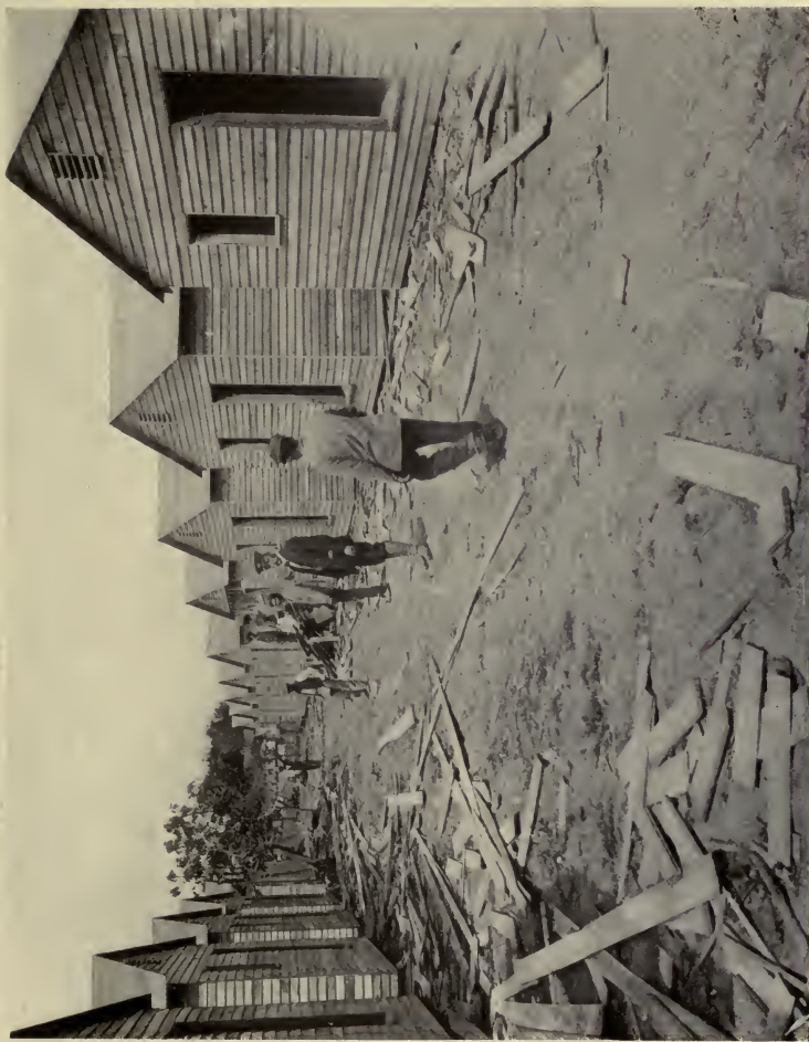
STREET OF HOUSES AFTER THE "ENCLOSERS" HAD FINISHED The Superintendent Carpenter in the middle is Mr. Neill Mackay who superintended fifty enclosing gangs of four men each.
