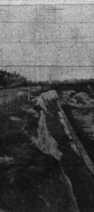
WASTING OF DALLAS ROAD FORESHORE.
